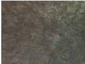
Steel surface largely covered with adhering mill scale but little, if any, rust.
