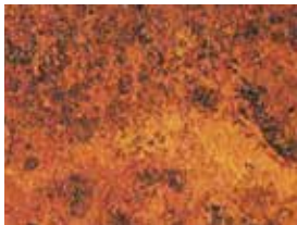
Mill scale on steel surface has rusted away, general pitting is visible under normal vision.
