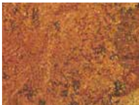
Mill scale on steel surface has rusted away, but with slight pitting visible under normal vision.
