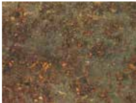
Steel surface has begun to rust and mill scale has begun to flake.
